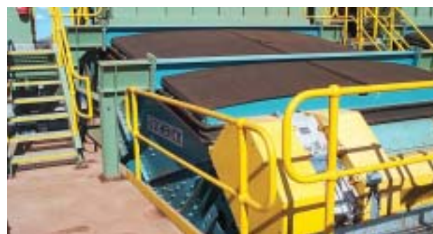
Banana screen dust enclosure
